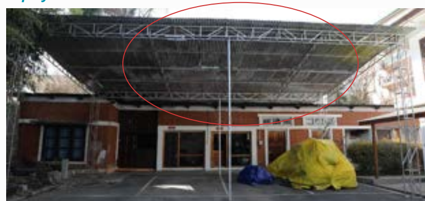
Portable multi-purpose utility shed setup at the HQ
