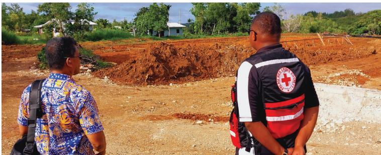
Chairman Santy Asanuma and Disaster Management Officer JB Victorino site visit to PRCS Lease in Ngebudel, Airai State. (for Emergency Storage Warehouse, 2023)
