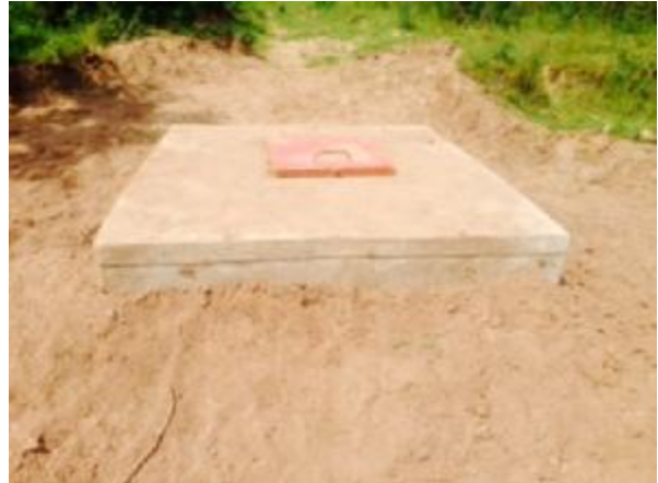
This is washout chamber
